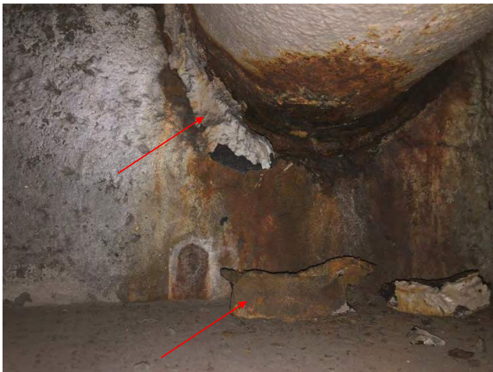
Photo 6 – View of the degraded asbestos-containing packing/sealant associated with the gas utility conduit at the west abutment of BIN 1022630.
