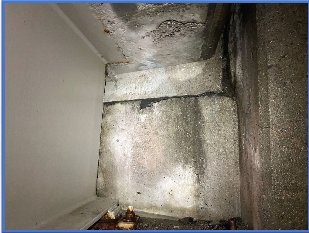
Photo 7 - Compressed asbestos sheet packing located on the abutment shelves at BIN 1022630 was confirmed as an ACM. Picture taken at the southeast quadrant of the bridge.
