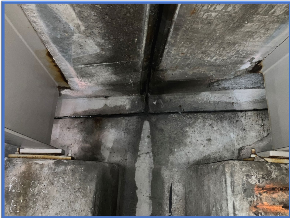
Photo 8 - Compressed asbestos sheet packing located on the abutment shelves at BIN 1022630 was confirmed as an ACM. Picture taken at the center of the east abutment.
