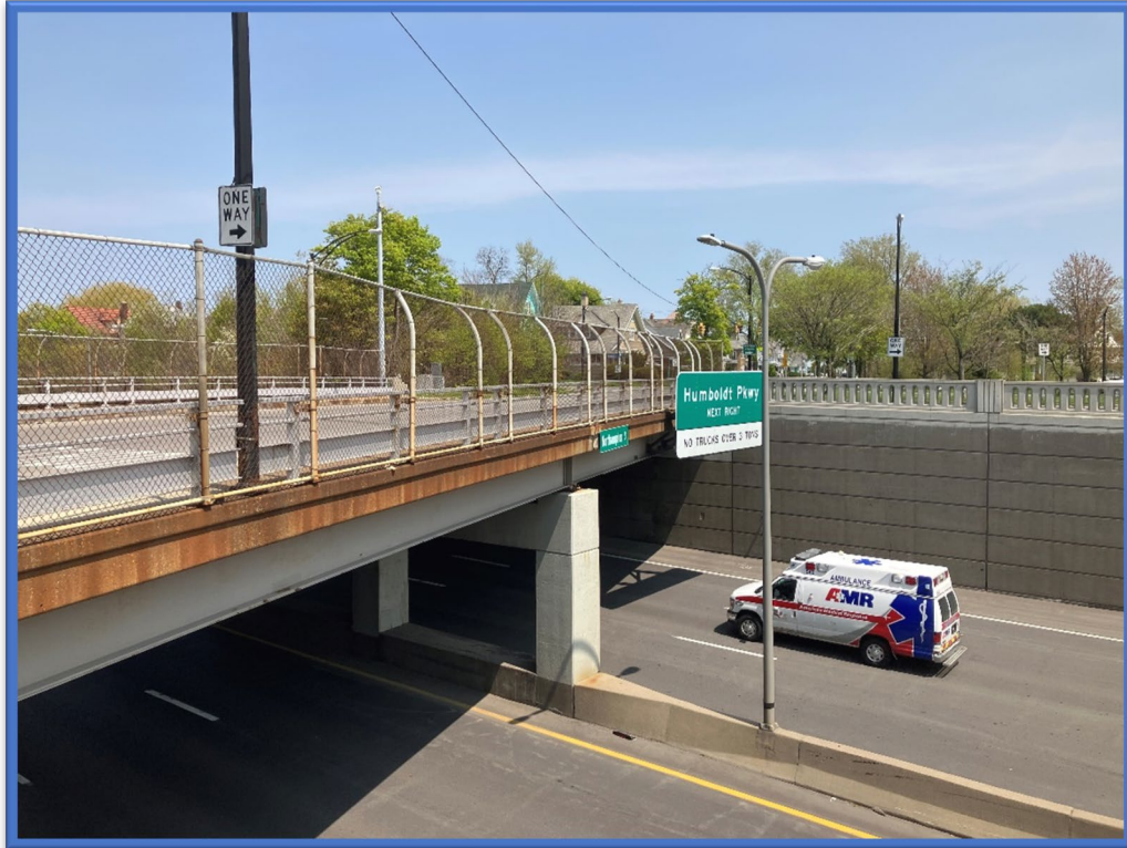
Photo 1 - View to the southern side of the Northampton Street Bridge over Kensington Expressway (Route 33) (BIN 1022620).
