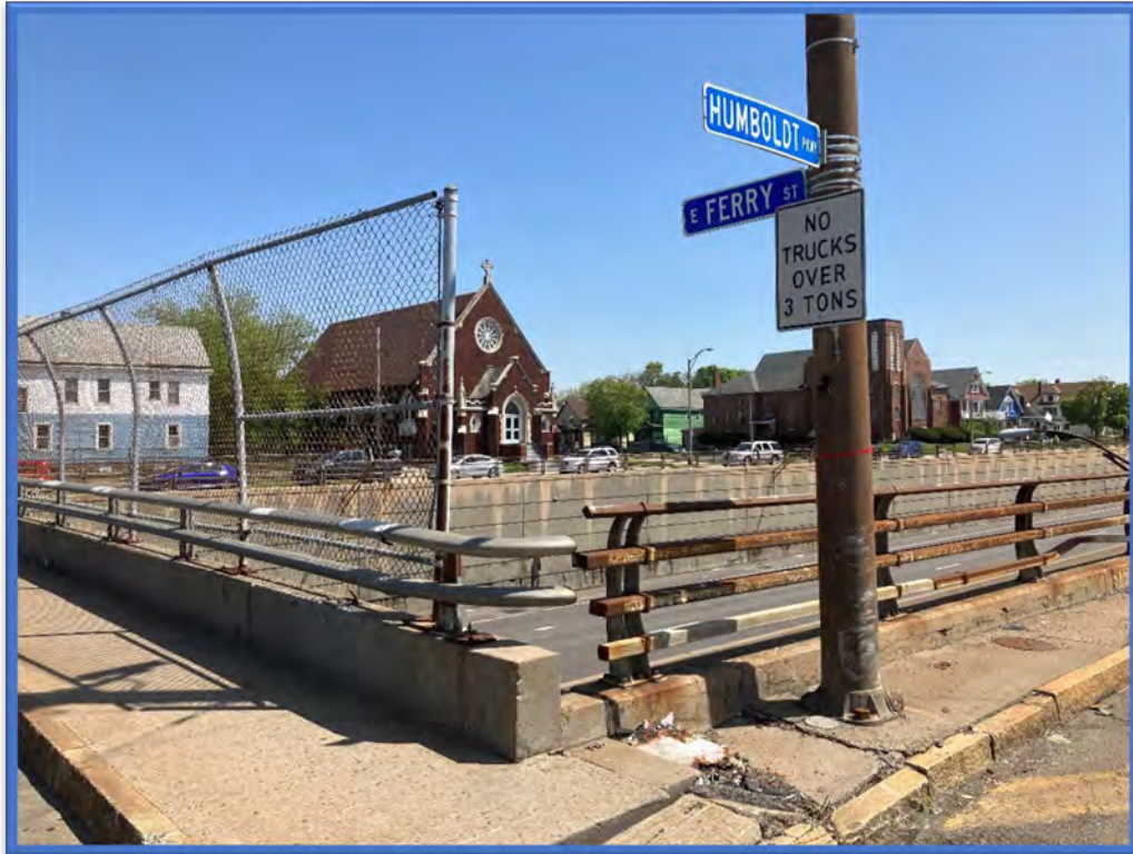
Photo 1 - View towards the southeast of the E Ferry Street Bridge over Kensington Expressway (Route 33) (BIN 1022640). The retaining wall ACMs (expansion joint caulking and railing post caulking) are visible within the photo.
