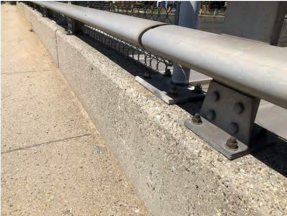
Photo 10 – View of the curb/knee wall along the north side of BIN 1022630. No ACM was identified in association with the associated concrete expansion joint caulk, guide rail, or fence posts.
