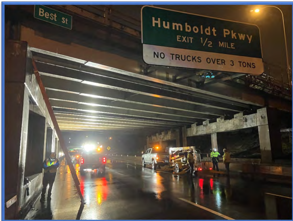
Photo 6 – View looking south towards the northeast side of BIN 1022609 during the night-time inspection that occurred after closing the EB Kensington Expressway (EB Route 33).
