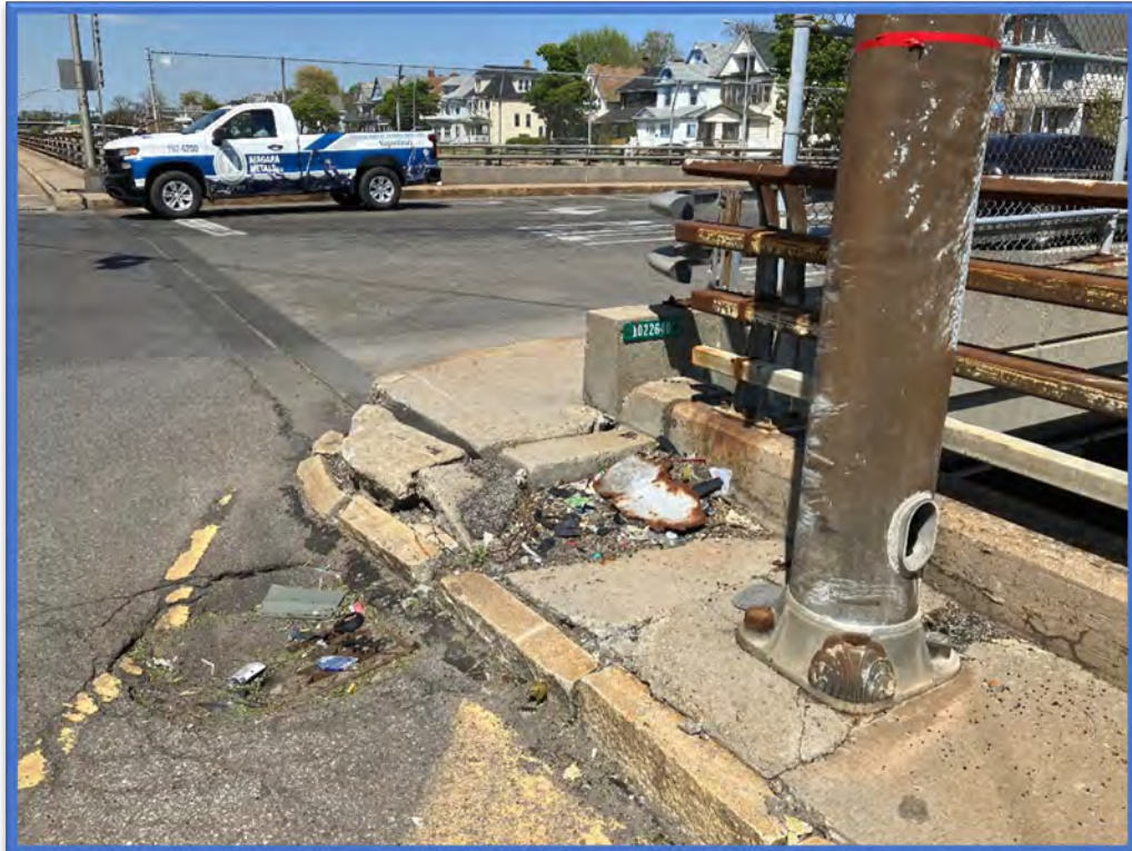
Photo 2 - View of the BIN plate located at the southwest corner of the E Ferry Street Bridge over Kensington Expressway (Route 33) (BIN 1022640).
