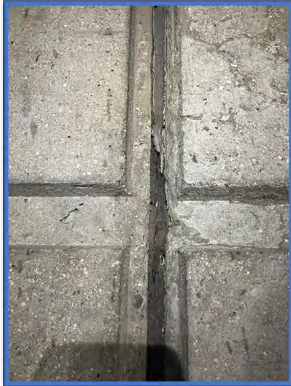
Photo 7 – View of the dark grey asbestos-containing caulking observed within the expansion joint at the Dodge Street Bridge over Kensington Expressway (Route 33) (BIN 1022610).
