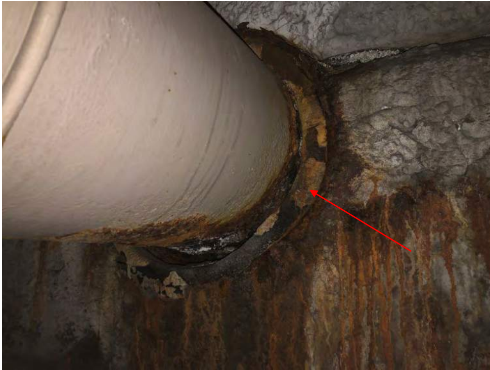
Photo 5 – View of the 12” metal conduit associated with the 8” gas utility line where it penetrates the east abutment of BIN 1022630. The packing/sealant around the perimeter of the 12” conduit where it penetrates each abutment has been identified as an ACM.
