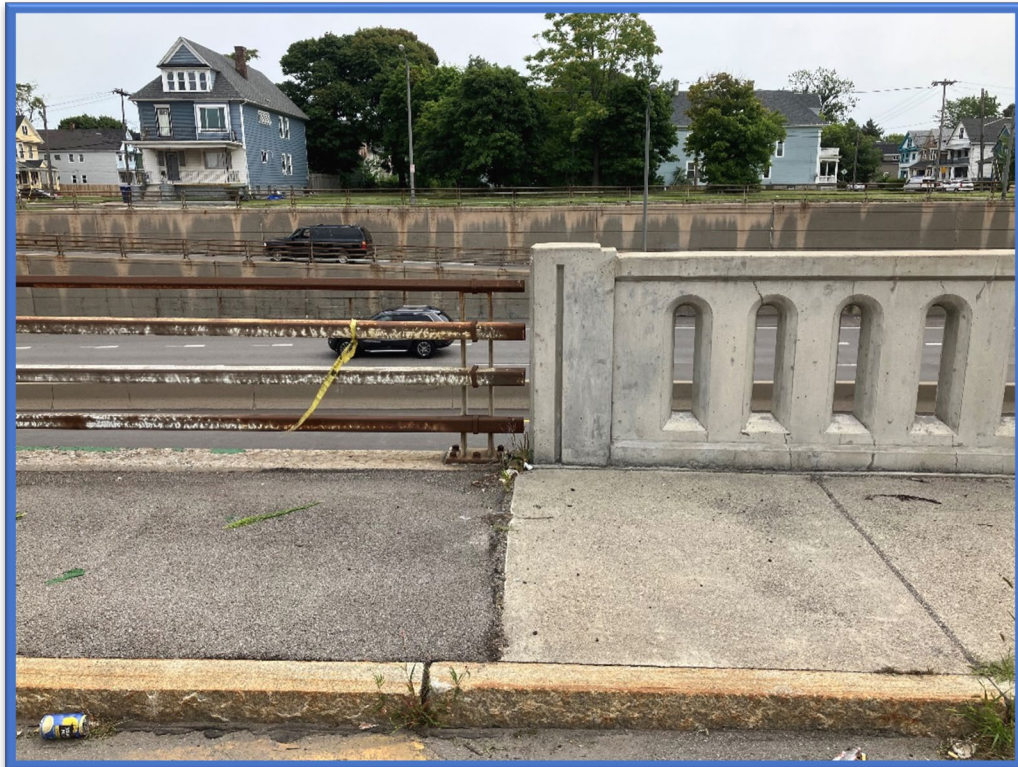
Photo 9 – Asbestos-containing railing post base caulk is associated with all of the metal guiderails located on top of the northern retaining walls. No asbestos-containing caulk is associated with the new decorative concrete guide rails located on top of the southern retaining walls.
