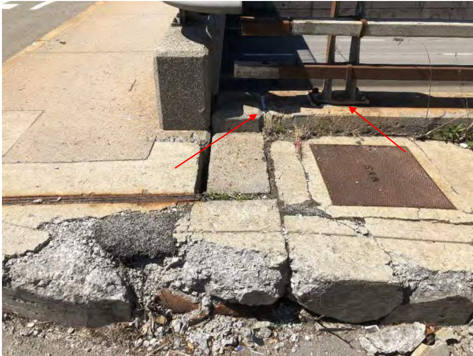
Photo 9 – View facing west at the northeast corner of BIN 1022630 and the retaining wall. The retaining wall grey caulk and the retaining wall guide rail post grey caulk have both been identified as an ACM. The retaining wall caulk is located along the vertical and horizontal face of the retaining wall.
