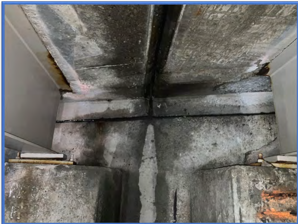
Photo 8 - Compressed asbestos sheet packing located on the abutment shelves at BIN 1022609 was confirmed as an ACM. Picture taken at the center of the east abutment.
