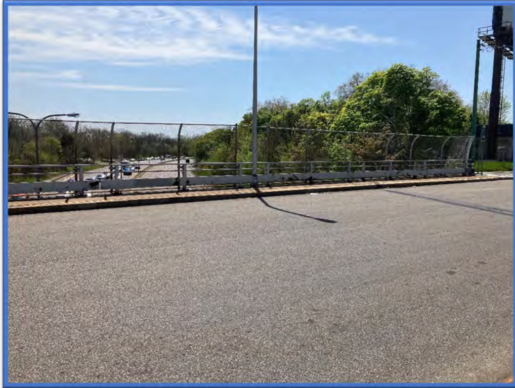
Photo 3 - View to the south from the middle of the Best Street Bridge over Kensington Expressway (Route 33) (BIN 1022609).
