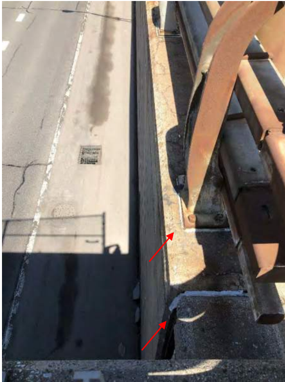
Photo 8 – View facing north at the northeast corner of BIN 1022630 and the retaining wall. The retaining wall grey caulk and the retaining wall guide rail post base grey caulk have both been identified as an ACM.
