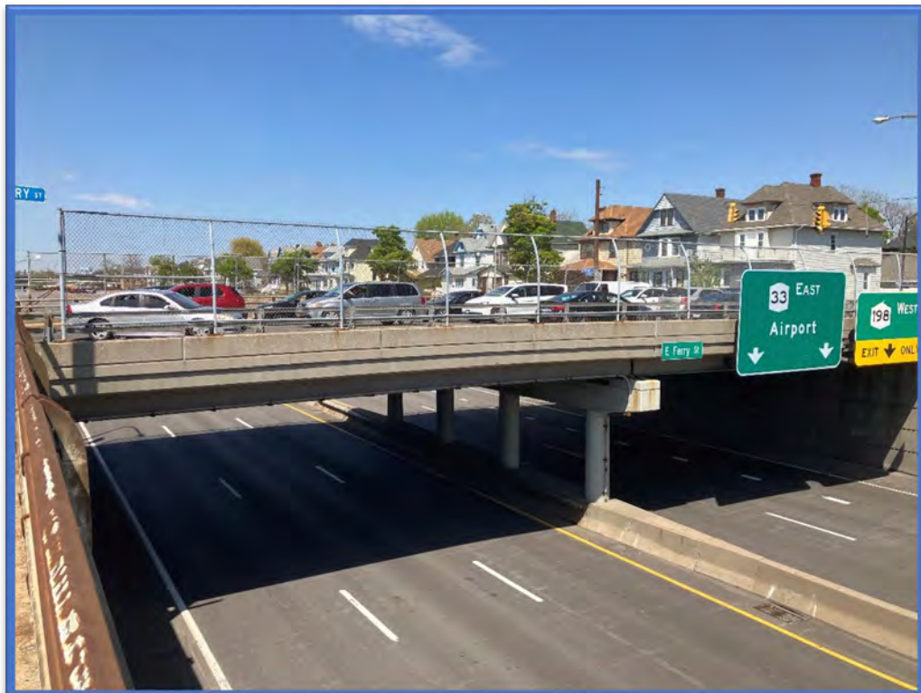
Photo 4 - View to the southern side of the E Ferry Street Bridge over Kensington Expressway (Route 33) (BIN 1022640).
