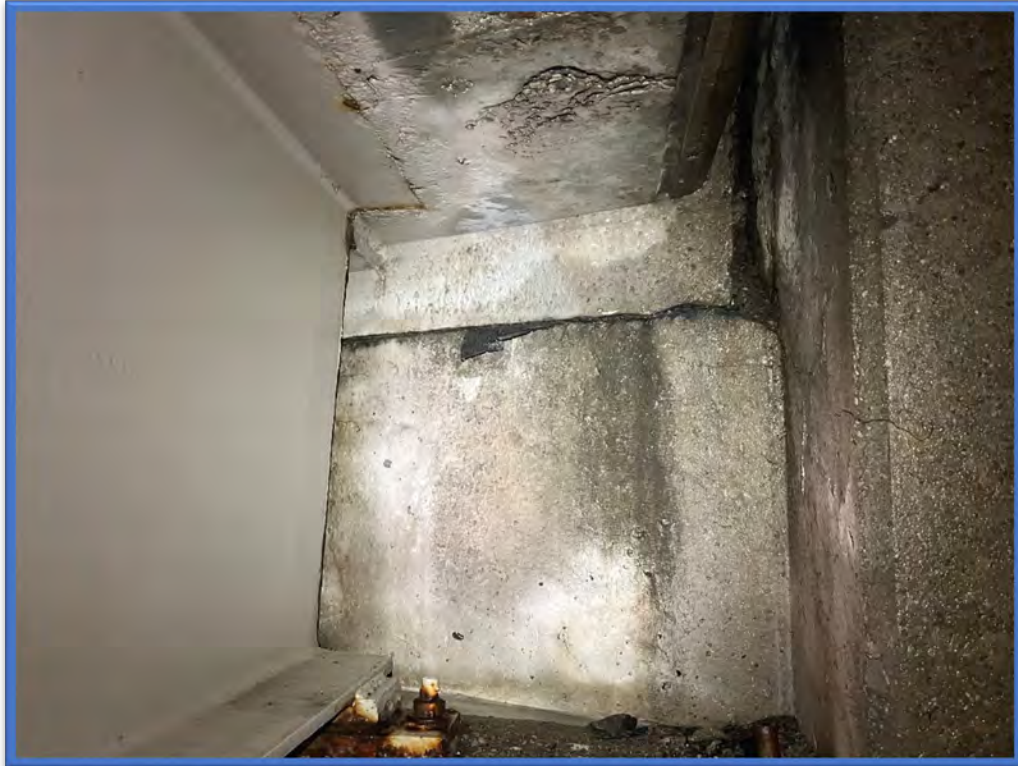
Photo 7 - Compressed asbestos sheet packing located on the abutment shelves at BIN 1022609 was confirmed as an ACM. Picture taken at the southeast quadrant of the bridge.
