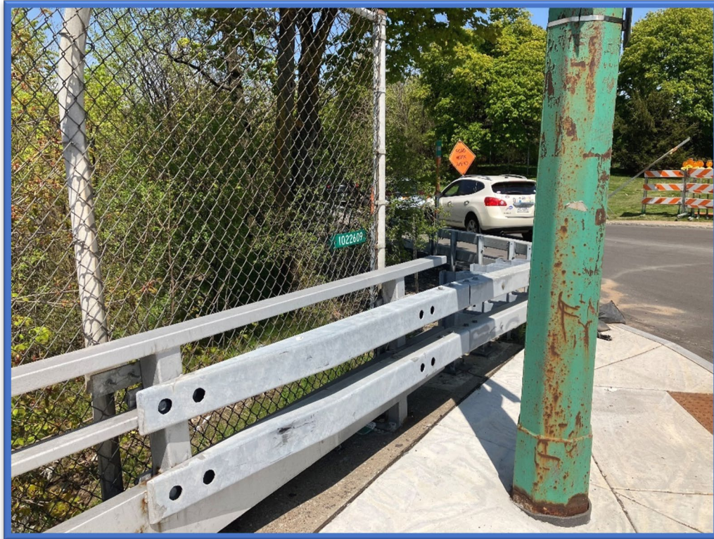
Photo 5 – BIN plate located on the adjacent fence at the northeast quadrant of BIN 1022630.
