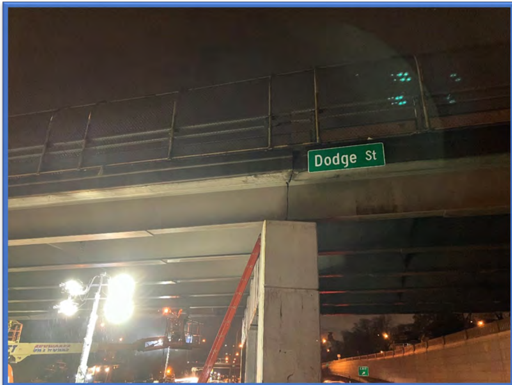
Photo 6 – View of the underside of the Dodge Street Bridge over Kensington Expressway (Route 33) (BIN 1022610) taken during the night-time inspection of the bridge.
