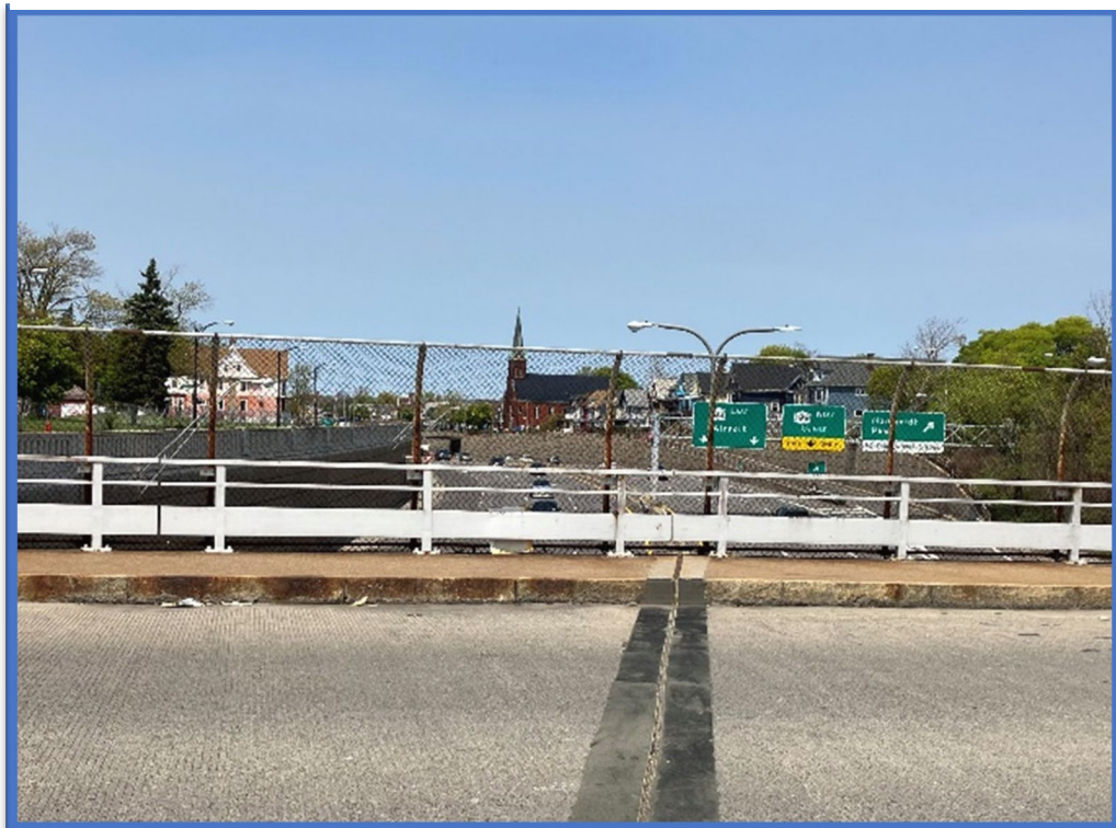
Photo 2 - View to the north from the middle of the deck of the Northampton Street Bridge over Kensington Expressway (Route 33) (BIN 1022620). Project corridor retaining walls are visible in the background of the photo.
