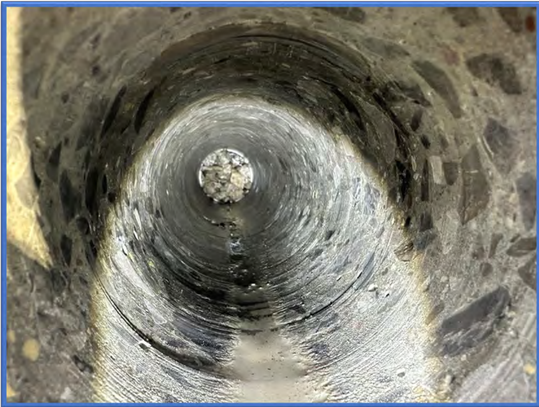
Photo 6 – Inside of the retaining wall core hole with stone visible on the back side.
