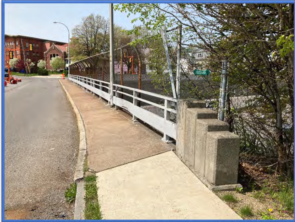
Photo 1 - View to the northwest of the northern side Dodge Street Bridge over Kensington Expressway (Route 33) (BIN 1022610).
