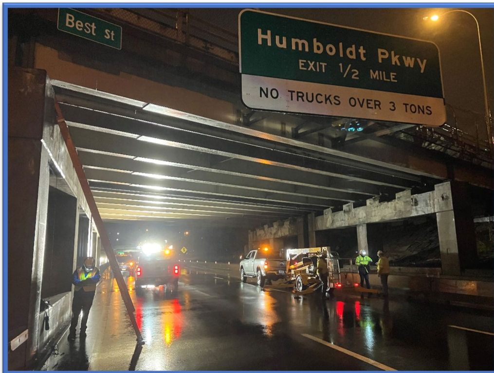
Photo 6 – View looking south towards the northeast side of BIN 1022630 during the night-time inspection that occurred after closing the EB Kensington Expressway (EB Route 33).
