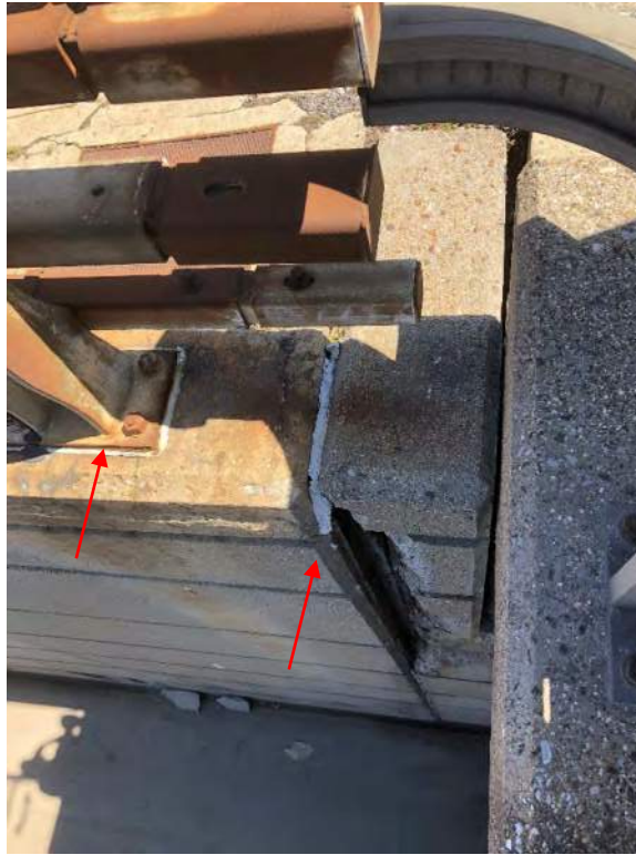
Photo 7 – View facing east at the northeast corner of BIN 1022630 and the retaining wall. The retaining wall grey caulk and the retaining wall guide rail post base grey caulk have both been identified as an ACM. The retaining wall caulk is degraded in places.
